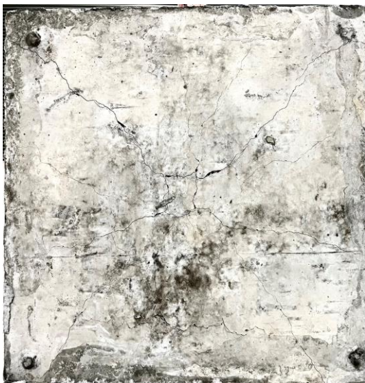
Fig. 9 Bottom surface crack patterns at failure of F2
