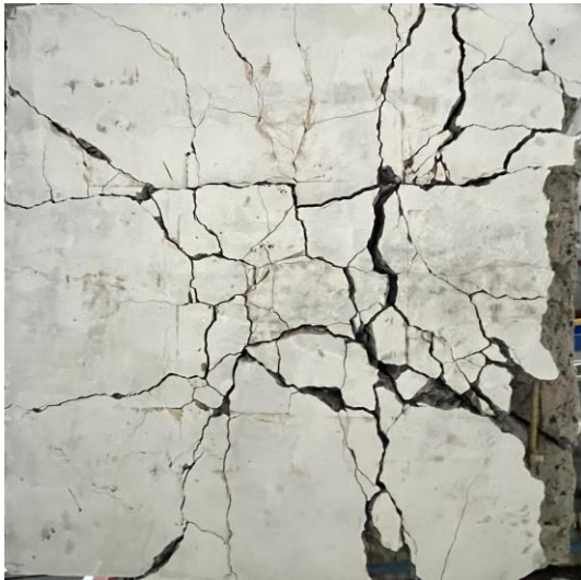
Fig. 8 Bottom surface crack patterns at failure of F1
