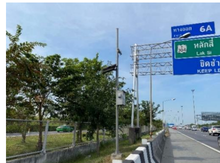
Fig. 4 The example of microwave sensor installation
