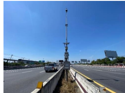
Fig. 3 The installation of an image processing camera
