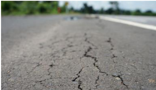
Fig. 3 Example of fatigue cracking
